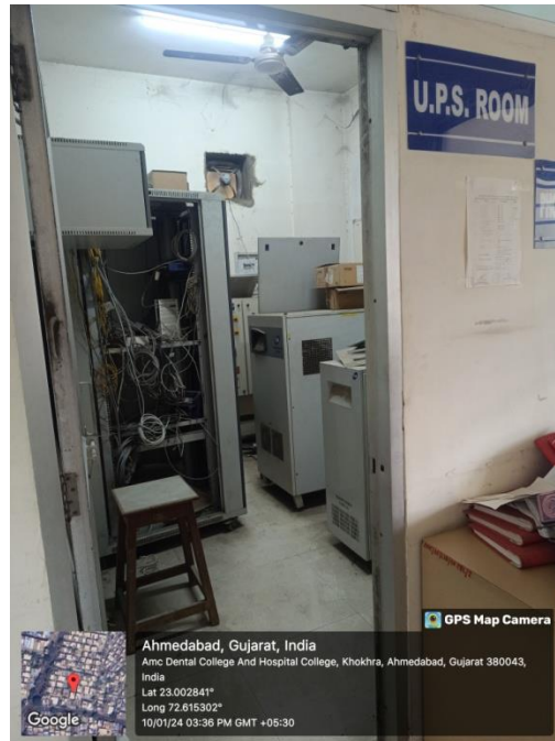
UPS located in the server room inside the library, located at first floor of college Building
