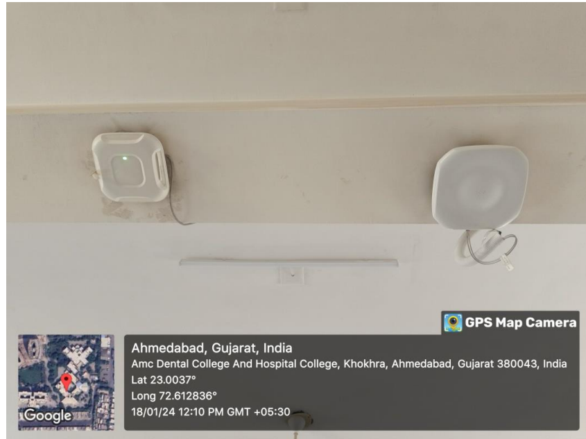
WiFi Router in the Orthodontics Preclinical Lab located at second floor of College Building
