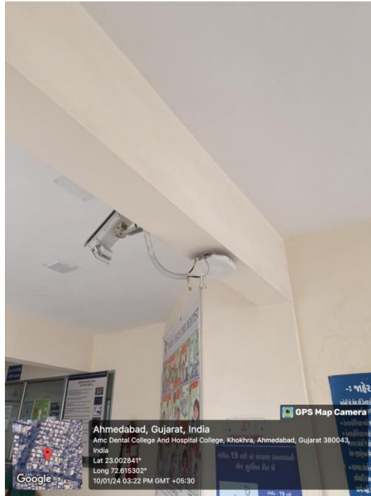
WiFi Router in the Paediatrics clinical area located at third floor of Hospital Building
